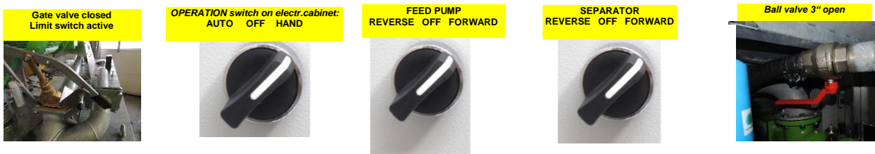
Figure 22 lever and switch position in manual operation with clear effluent pump
