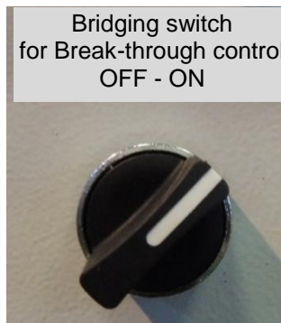
Figure 11 Bridging switch for break through control
